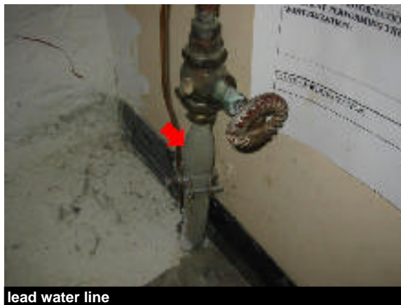
lead water line
