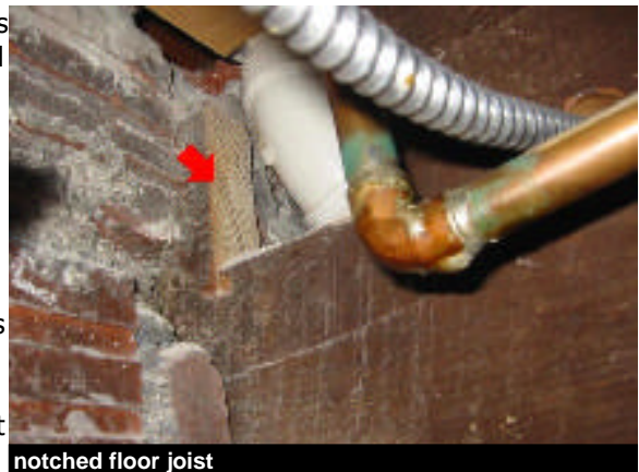
notched floor joist
