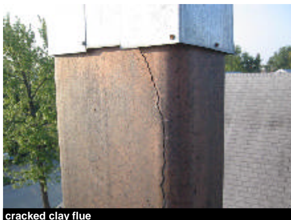
cracked clay flue
