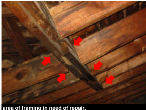
area of framing in need of repair.
