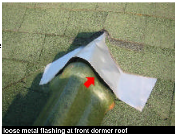
loose metal flashing at front dormer roof
