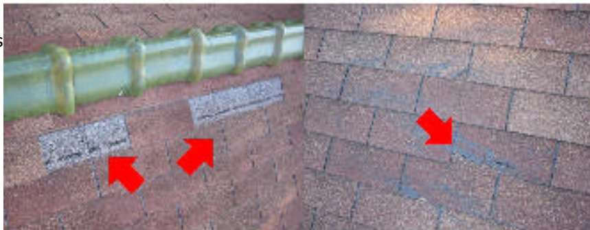
missing shingles / worn areas
